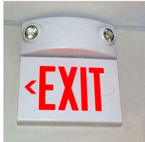
Figure 42: Emergency Dual Beam Lighting
