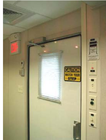
Staff Entry Door Controls
