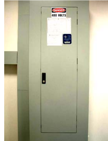
Figure 27: 480V AC Electrical Panel (interior)
