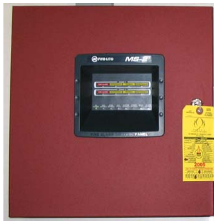
Figure 18: Fire Alarm Control Panel
