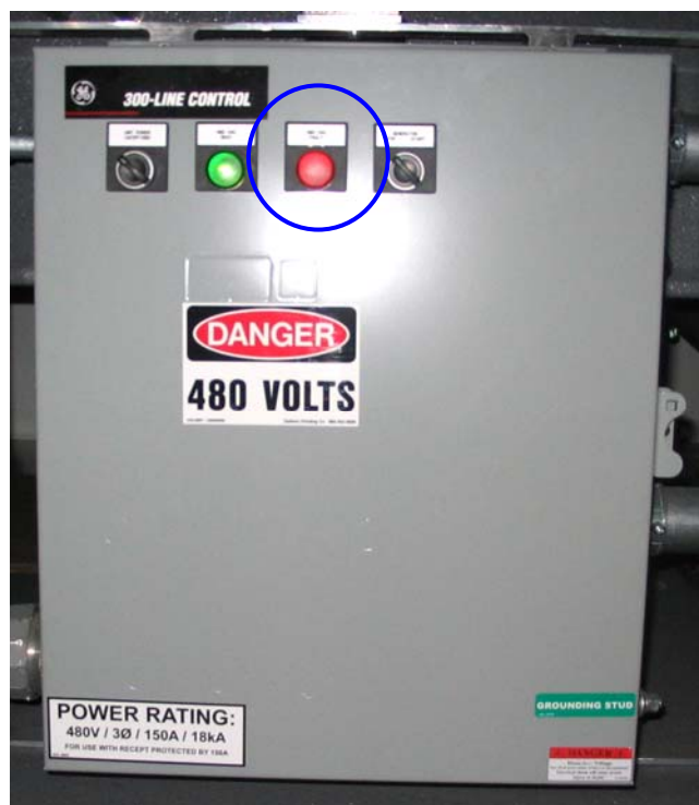
Figure 47: 480V AC Fault Indicator Light
