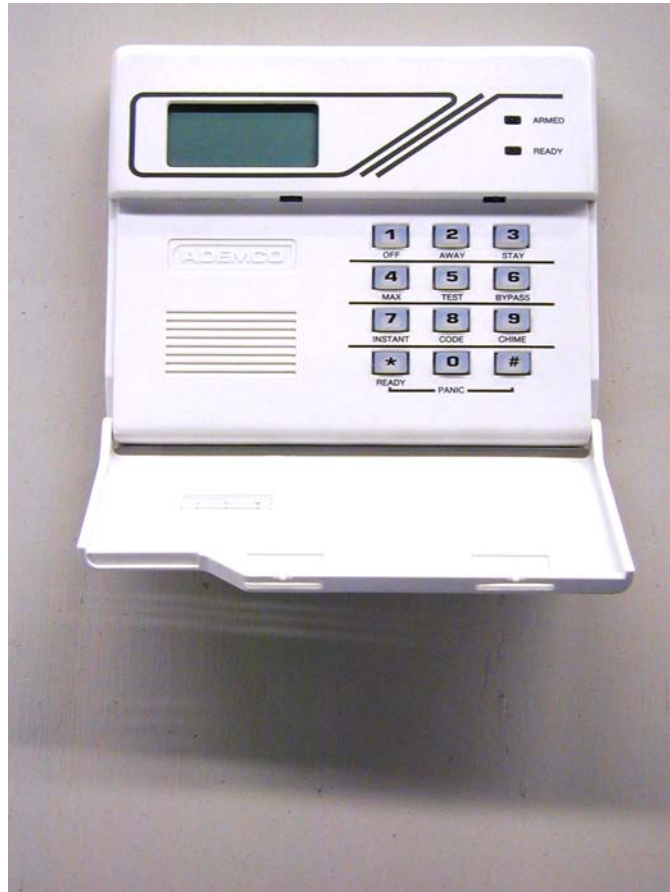
Figure 38: Intrusion Alarm Keypad
