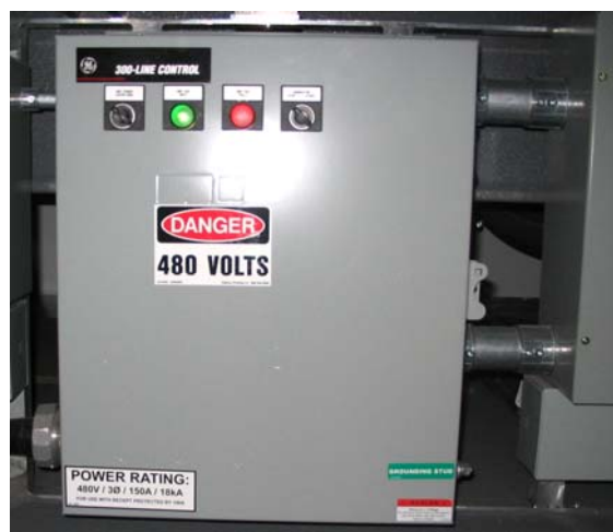
Figure 25: 480V AC Electrical Control Panel
