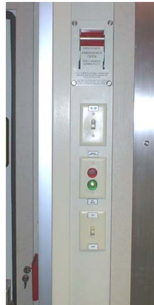
Figure 11 Mobile Unit Controls
