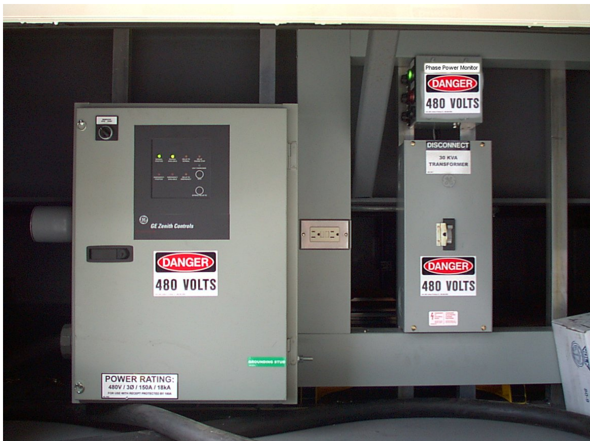
Figure 29: 480V AC ATS and Phase Power Monitor
