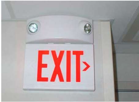
Control Room Emergency Light
