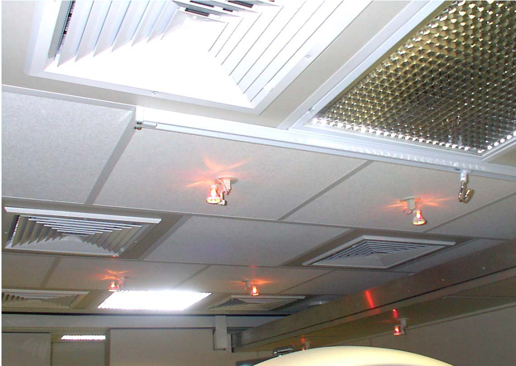
Figure 50: Gantry Room Overall Lighting
