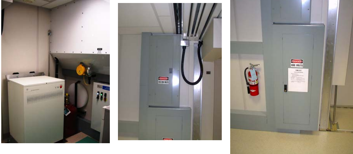
Figure 28: 480V and 120/208V AC Electrical Panels
