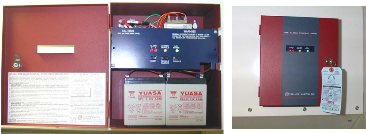
Figure 19: Fire Alarm Control Panel
