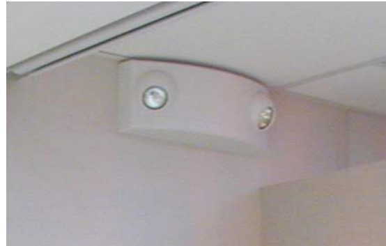
Gantry Room Emergency Light
