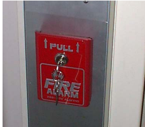
Figure 20: Fire Alarm Pull Station
