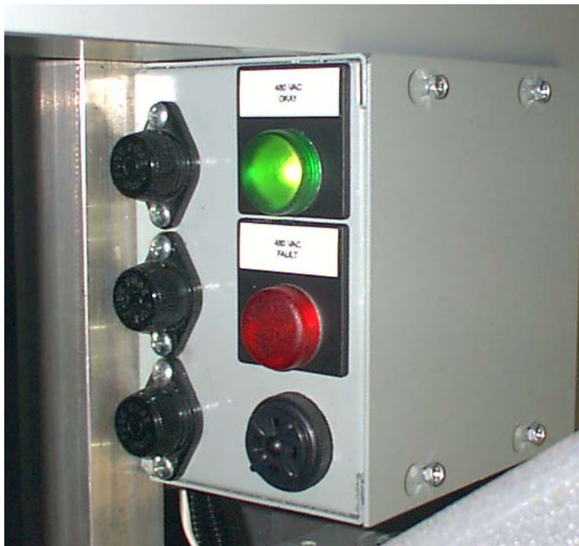
Figure 30: 480V AC Phase Power Monitor
