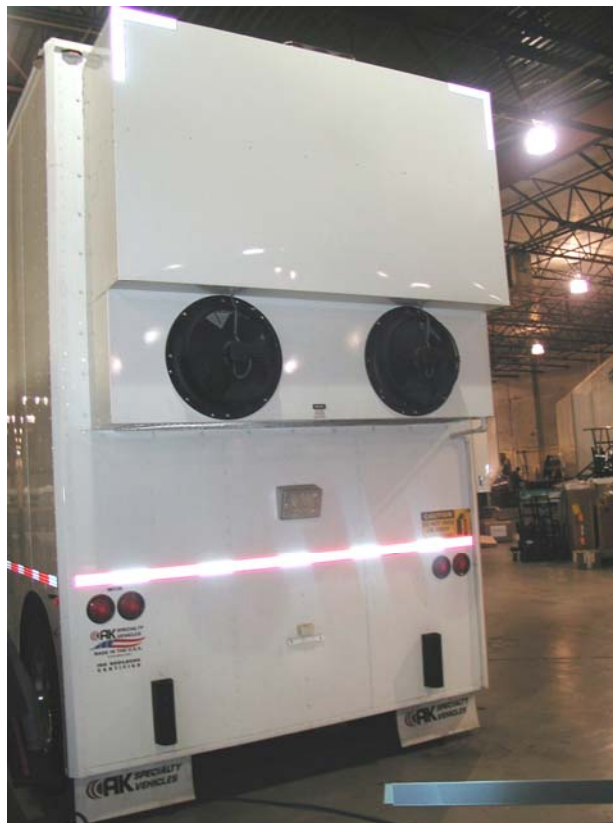
Figure 38: Northern Air A/C Units
