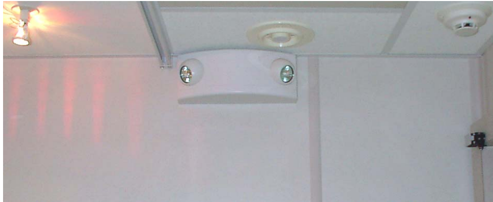
Dispensing Room Emergency Light
