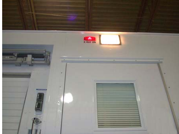
Figure 48: Staff Door Lighting
