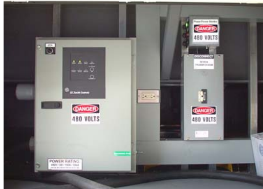
Figure 26: Automatic Transfer Switch and Phase Power Monitor
