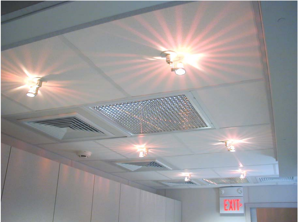
Figure 49: Control Room Overall Lighting
