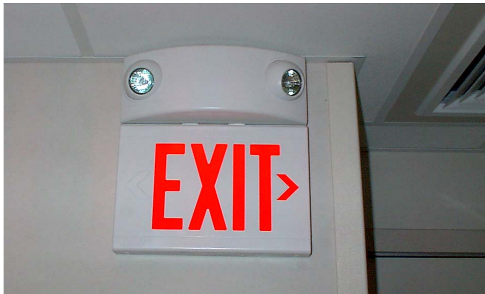
Figure 16: Control Room Emergency Lighting
